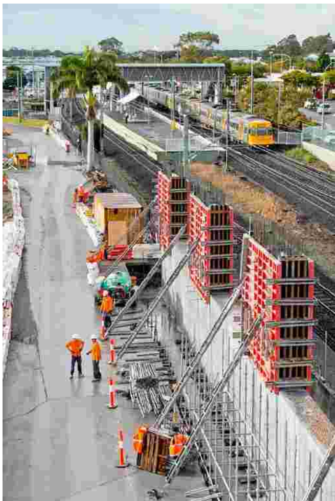
This photo of the construction of the Geebung overpass showing something of the massive concrete walls needed to stabilize the structure.
