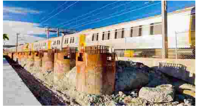
A photo of the construction of the new overpass at Geebung showing some of the construction on concrete pillars beside the existing train line
